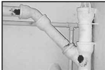
Rust on pipes or other parts of heating, plumbing or air conditioning equipment is also a sign of too much humidity.
