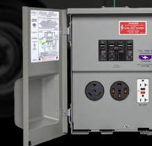
Shore Power / Generator
